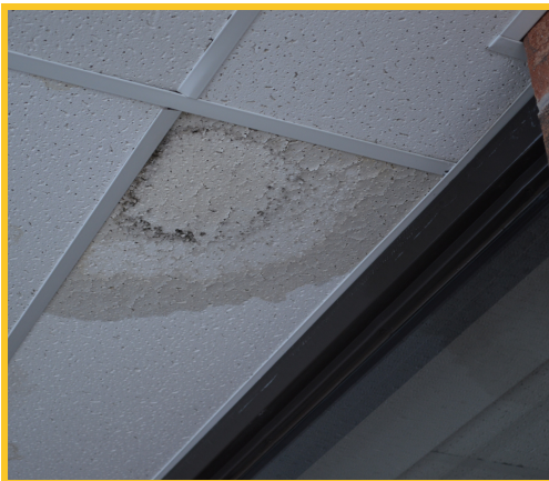
Evidence of roof leaks can be found inside several buildings.
