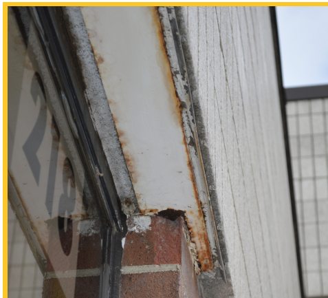
Repair damaged lintel at older single pane windows, which causes water and air infiltration issues.
