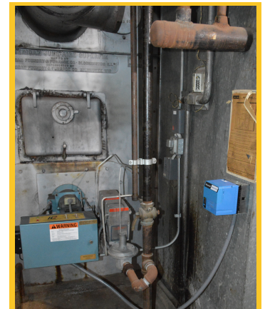
Aging equipment poses difficulties in obtaining parts prolonging and increasing costs of repairs.
